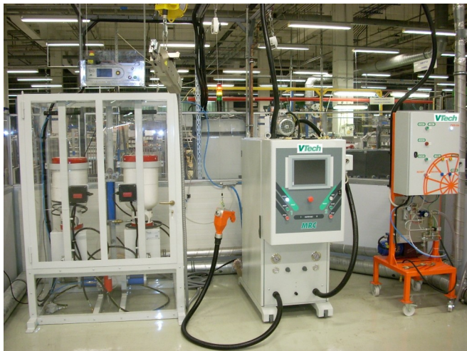
HC Installation including Supply, Charging and Purging
